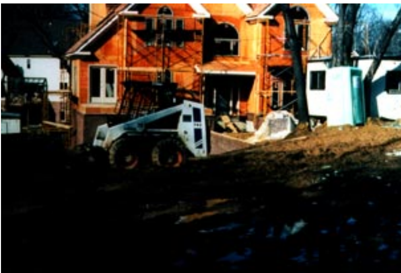
Figure 10 - The high erosion rate of construction sites is a major source of runoff from developing areas. Eroded materials contribute to siltation and eutrophication of lakes, rivers, and coastal oceans.
